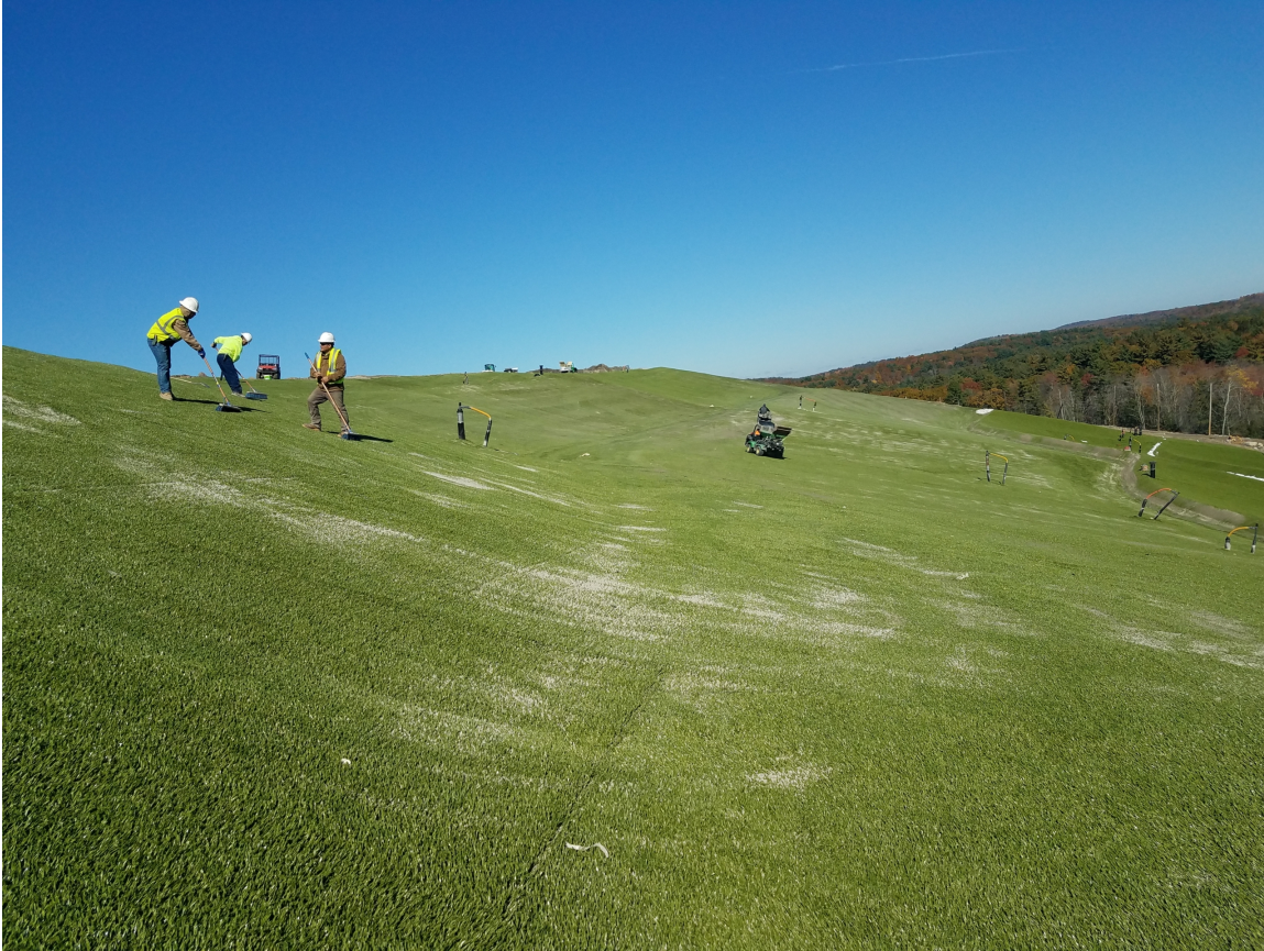
Image 1: Installation of ClosureTurf® system at the Southbridge Recycling & Disposal Park in Southbridge, MA.
