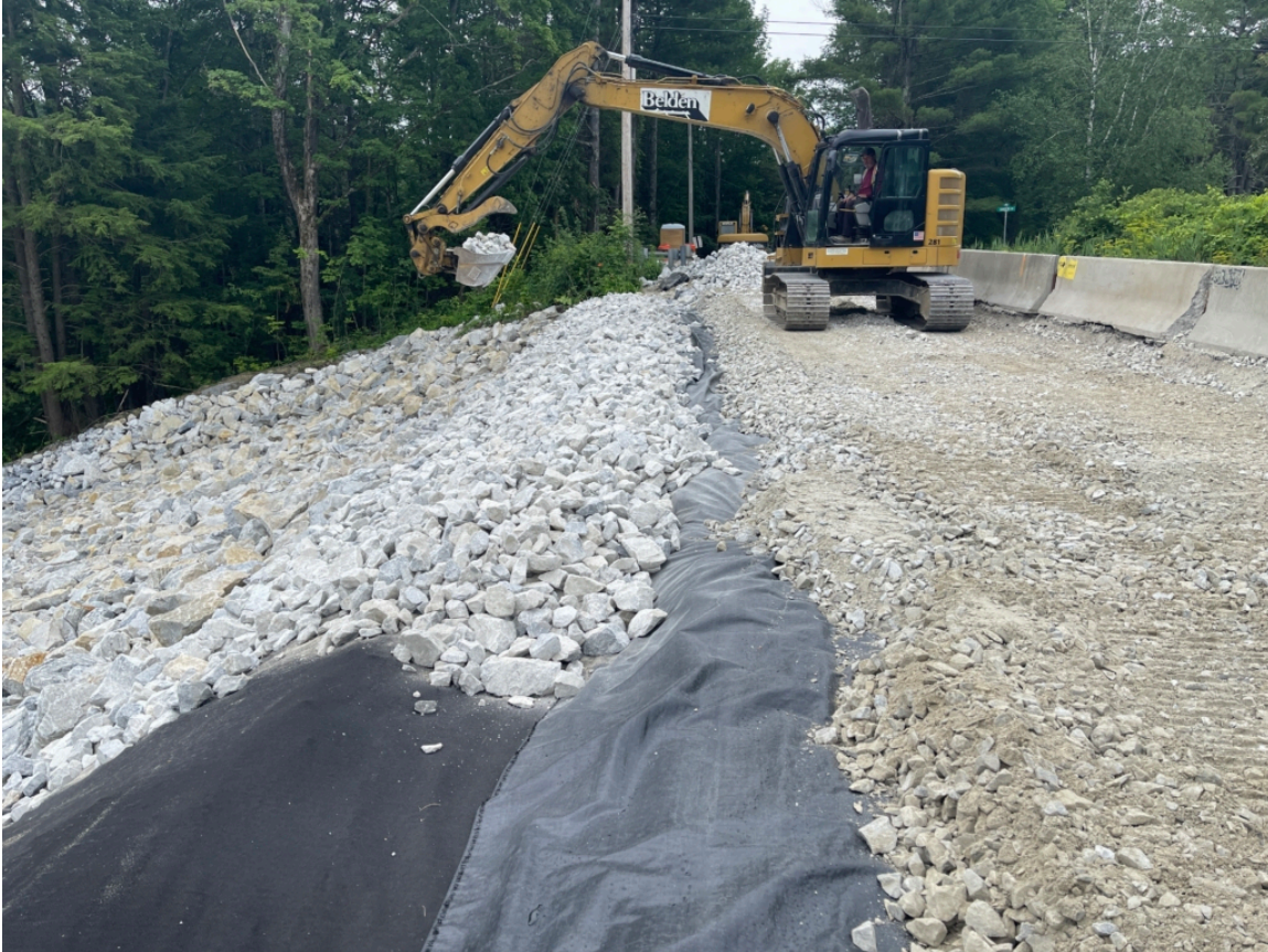
An example of a Level 3 resilient design is the reconstruction of Dewey Avenue in West Rutland, VT. Source: Sanborn, Head & Associates, Inc.
